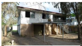
The Main family home. The water went nearly 3 metres over the roof
