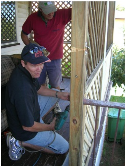
A care recipient's porch is being repaired by members of the Handyman Team of BPCC.
